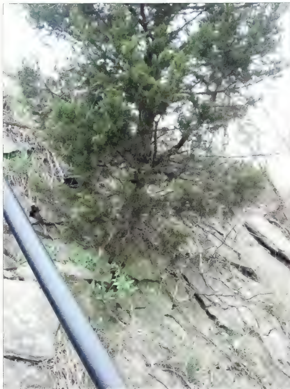
Figure 3.33. View looking east from access stairs, Battery Potter. The sloped portion of the concrete battery, rising approximately ten-feet above the engineered earthwork, has eastern red cedars ( Juniperus virginiana ) growing in cracks and in large spalling areas (Olmsted Center, April 2008).
